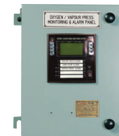
MONITORING & ALARM PANEL
