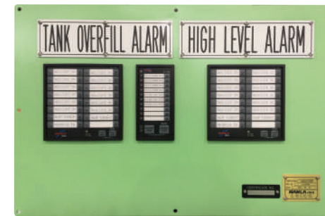
HIGH AND OVERFILL ALARM PANEL
