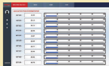
GAS DETECTOR MONITORING SENSOR VALUE AUDIO & VISUAL ALARM
